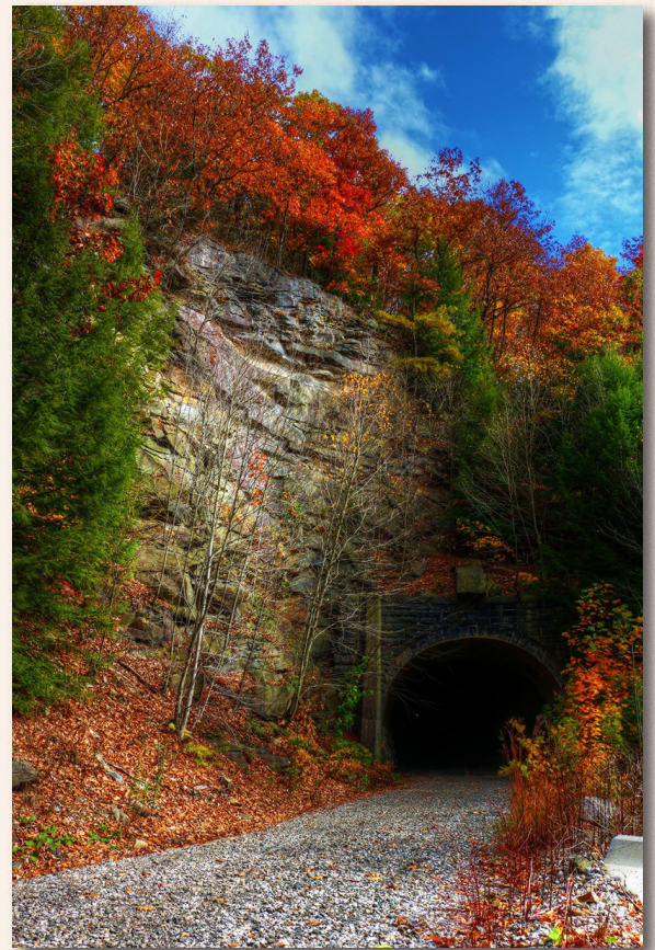
1872 Climax RR Tunnel, now part of the Redbank Valley Trail in Clarion County, is closed while work is done to repair and support the ceiling. Work on the tunnel will continue through 2016.
